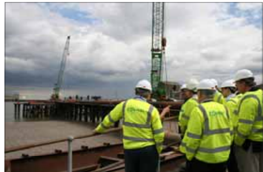
Refurbishing the pier and berth for ships to dock and unload material
